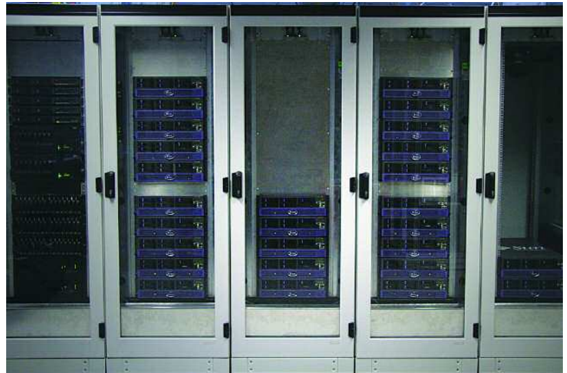
Figure 3: 64bit HPC Linux cluster with HA AIX file server in air-conditioned racks. The systems shown provide 112 CPUs, 872GB RAM and more than 25TB disk space
